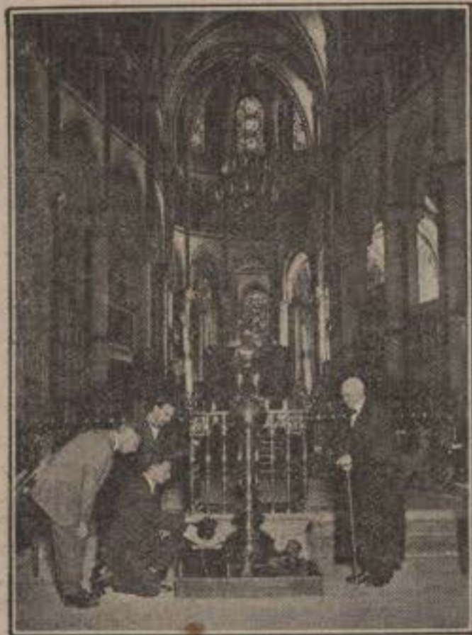
O.B. Engineers installing a microphone for the first broadcast from Canterbury Cathedral—an important transmission requiring special care.
